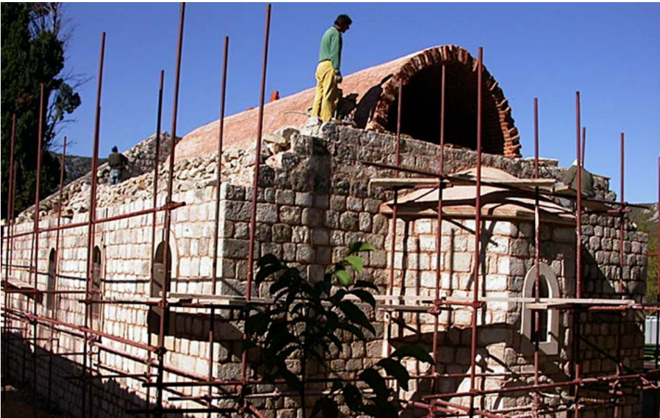
Fig. 16, Fig. 17. Reconstruction process at the site and remains of the 16 th C Eastern Orthodox Monastery in Žitomislići.
