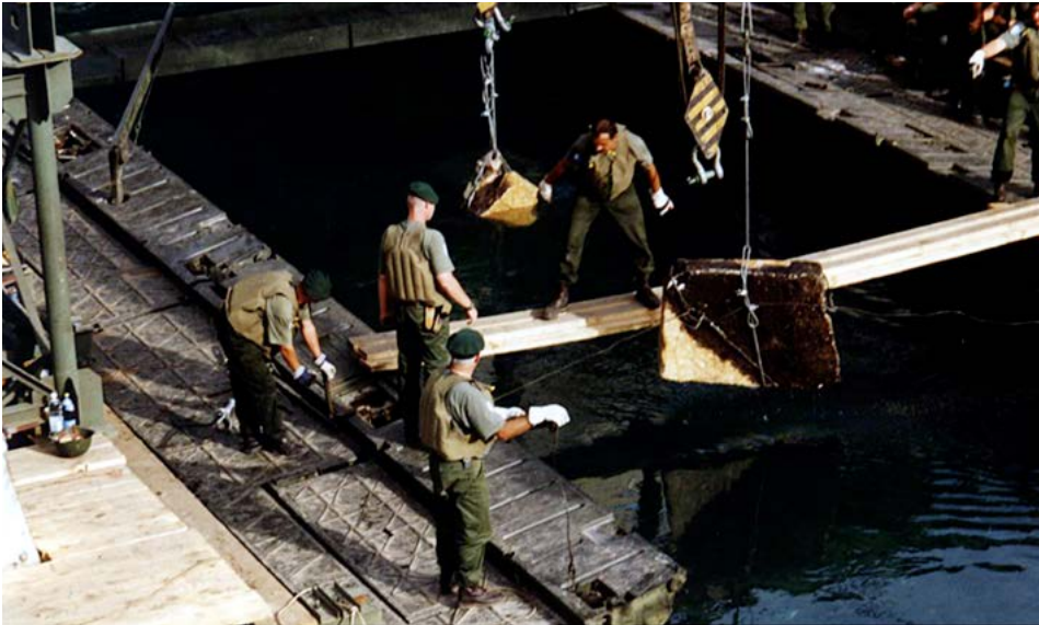
Fig. 11. Start of collecting fragments of the Old Bridge in Mostar from the river Neretva in 1997 (Photo: Sluejman Demirović).
