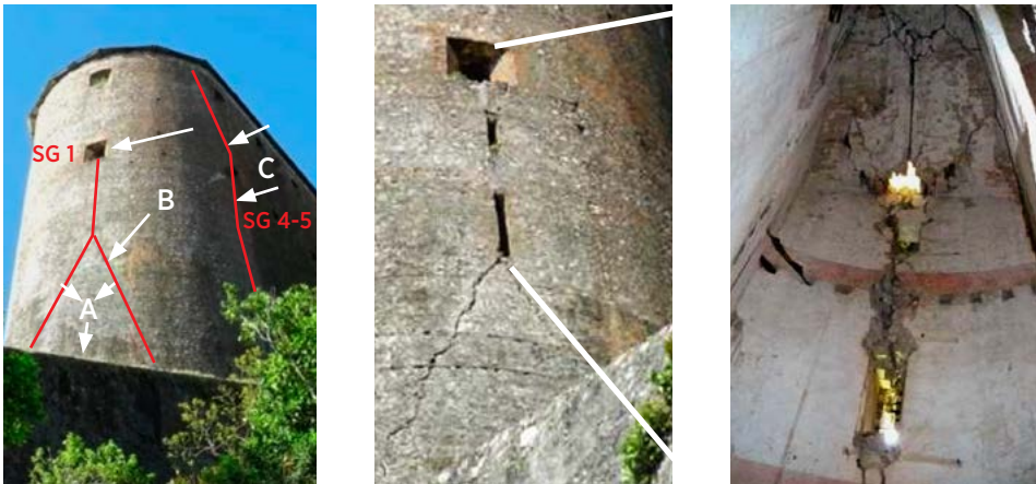
Fig. 11. View of ruptures on the axis of the windows, and the cracks of the Coidavid battery outside and inside.
