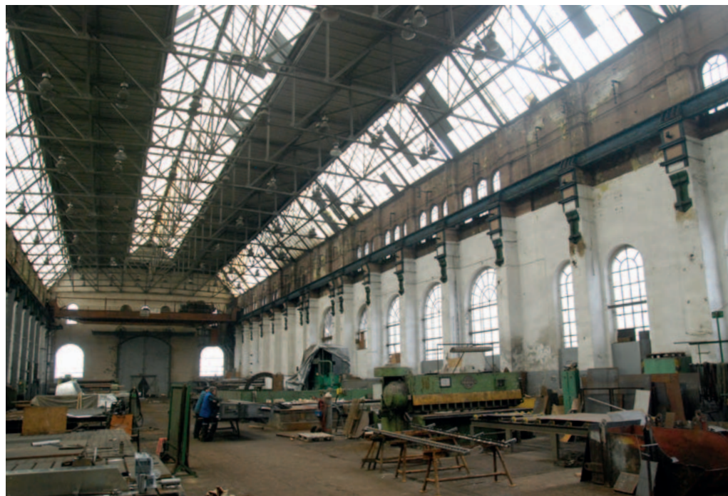
62. Interior of the machining hall. Attention is drawn to the skylights in the roof, providing good lighting for the workstations, the original semi-circular window openings and the crane beam laid on brick supports, 2021. Photo: A. Woźniakowski, collection of the author
