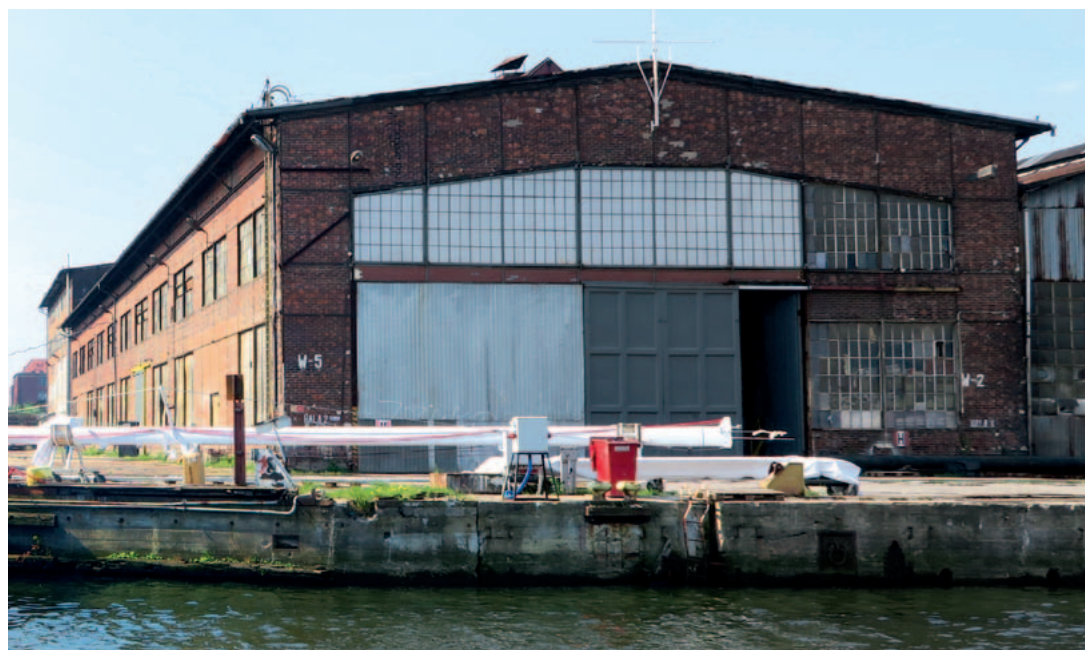
68. North elevation of boiler hall 2, 2018. Photo: T. Błyskosz, National Institute of Cultural Heritage archives
