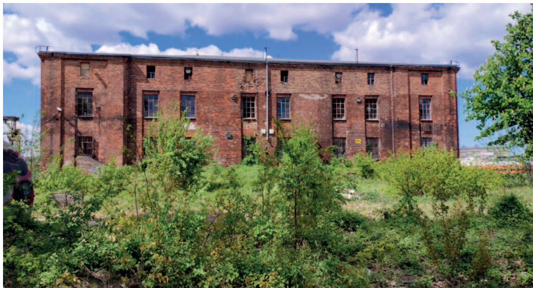
79. South elevation of the Gdańsk Shipyard furniture warehouse building (151A). The wall shows traces of numerous alterations and modernisations. The building is connected to an underground shelter, probably created during the Second World War. The shelter is located underground in the vegetated area visible in the foreground, 2022. Photo: A. Trzeciak, collection of the author
