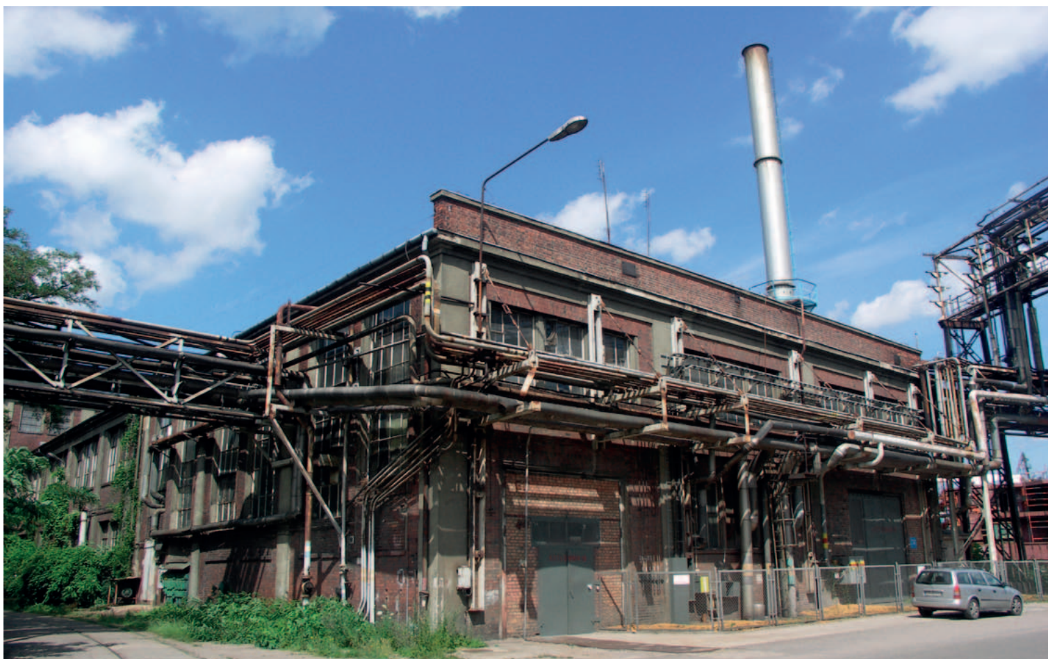
52. The hall of the shipyard boiler house with the now defunct overpasses with pipelines for the transmission of, among other things, industrial gases, 2009. Photo: T. Błyskosz, National Institute of Cultural Heritage archives
