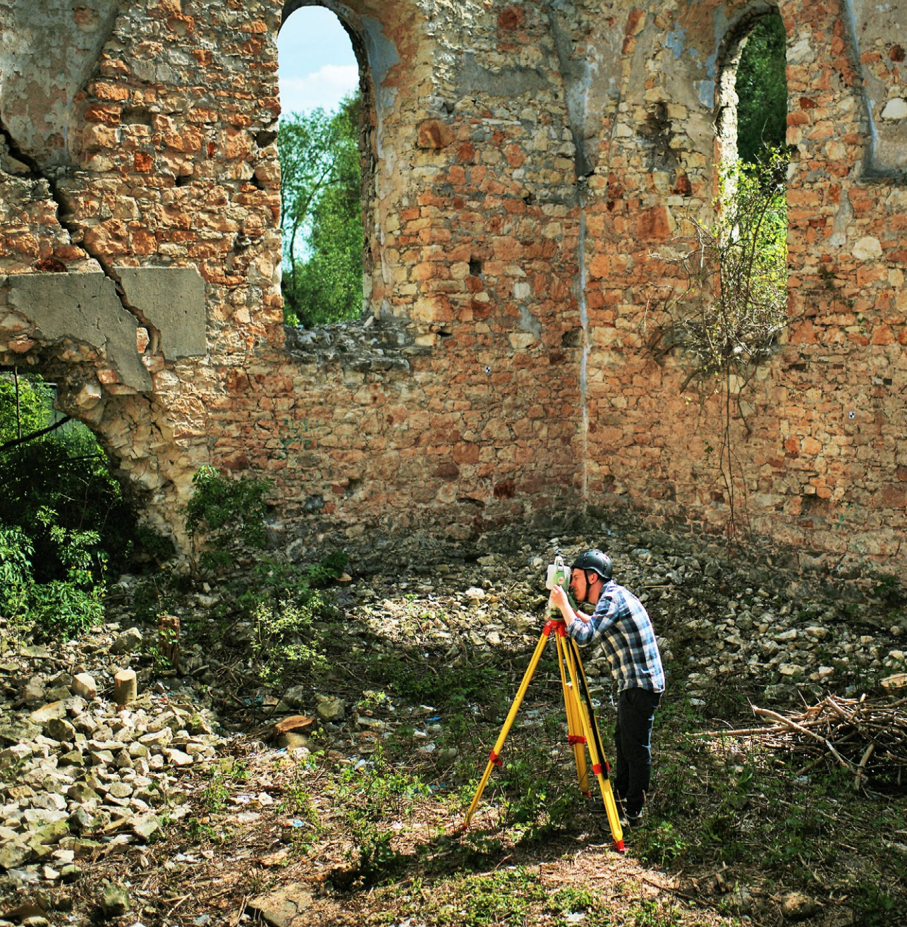
1 Tacheometric survey of the ruins of the synagogue in Tarłów (photo: K. Czajkowski)
